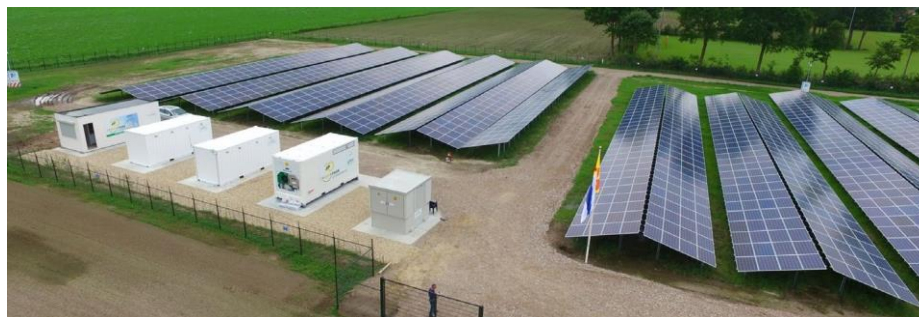
Energy storage at solar park Weert Energie
